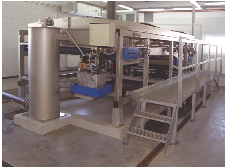
Sludge Belt Thickening Plant with hydraulically controlled Belt Thickener, Model ST, Waste Water Treatment Plant Legnica
